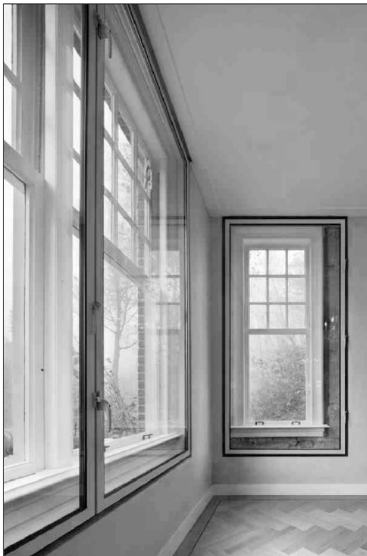
Figure 5: Example of an isolating material elements on the natural basis, compatible with conventional building techniques. Insulation by flax isolations with a clay plaster – Driebergen, the Netherlands
